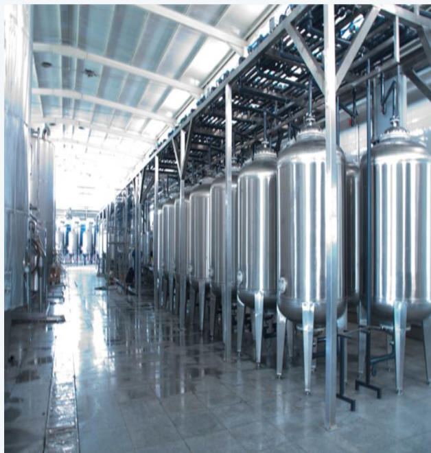
ION EXCHANGE SYSTEM
